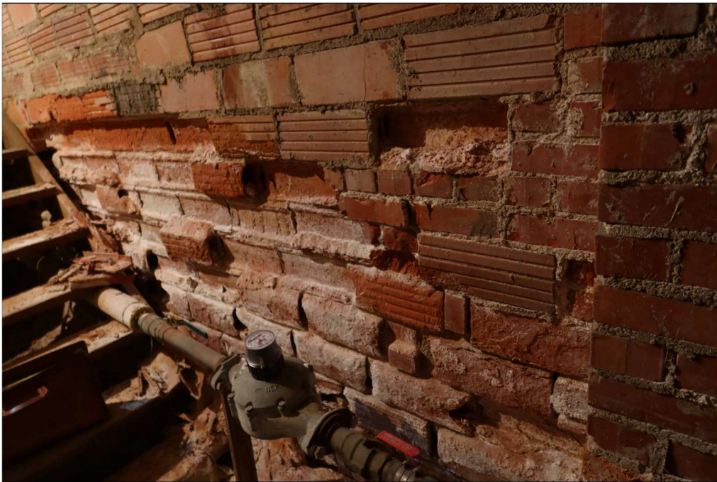
PICTURE 2 - DETERIORATED WALL
