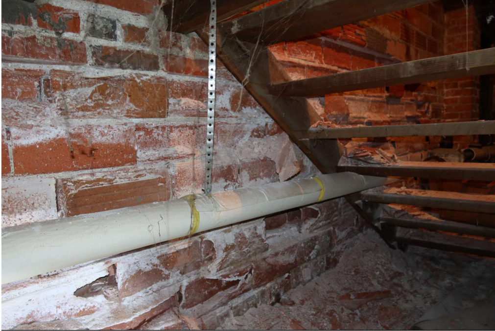
PICTURE 1 - DETERIORATED WALL
